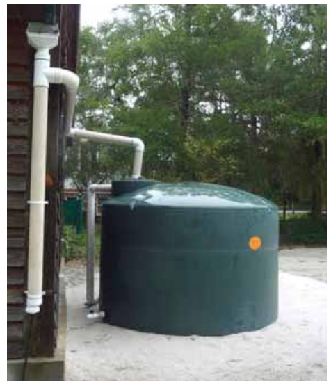
Cistern at DNR facility, Charleston.
