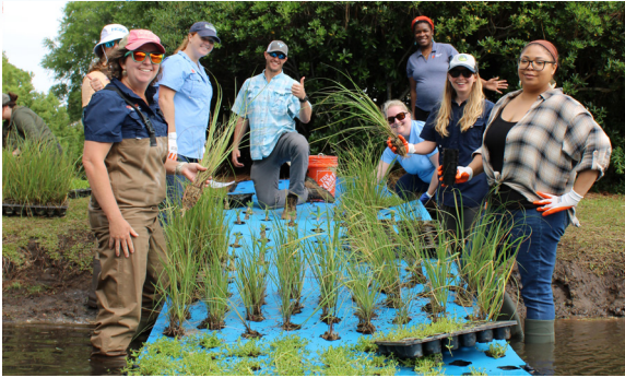
Floating Treatment Wetland install in Mount Pleasant. Thank you to our partners at the Town of Mount Pleasant.
