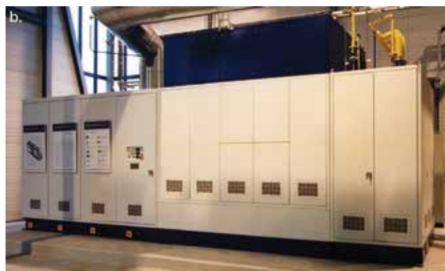
▲ Figure 3. (a) Siemens/Westinghouse has demonstrated a 220-kWe SOFC/micro-turbine hybrid generator that achieved a net electrical efficiency of 53%. (b) A different unit, a 100-kWe SOFC generator, has more than 35,000 hours of operation, making it the longest-running SOFC ever demonstrated. Source: Photos courtesy of Siemens/Westinghouse.
