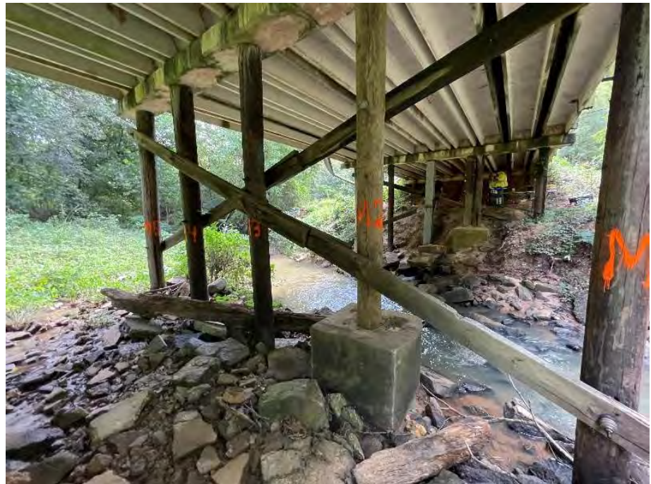
Timber piles supporting a bridge in Greenwood County, South Carolina. These piles were salvaged for research when the bridge was deconstructed and replaced.
